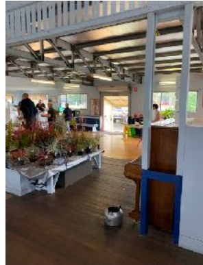
Even drips inside ...
